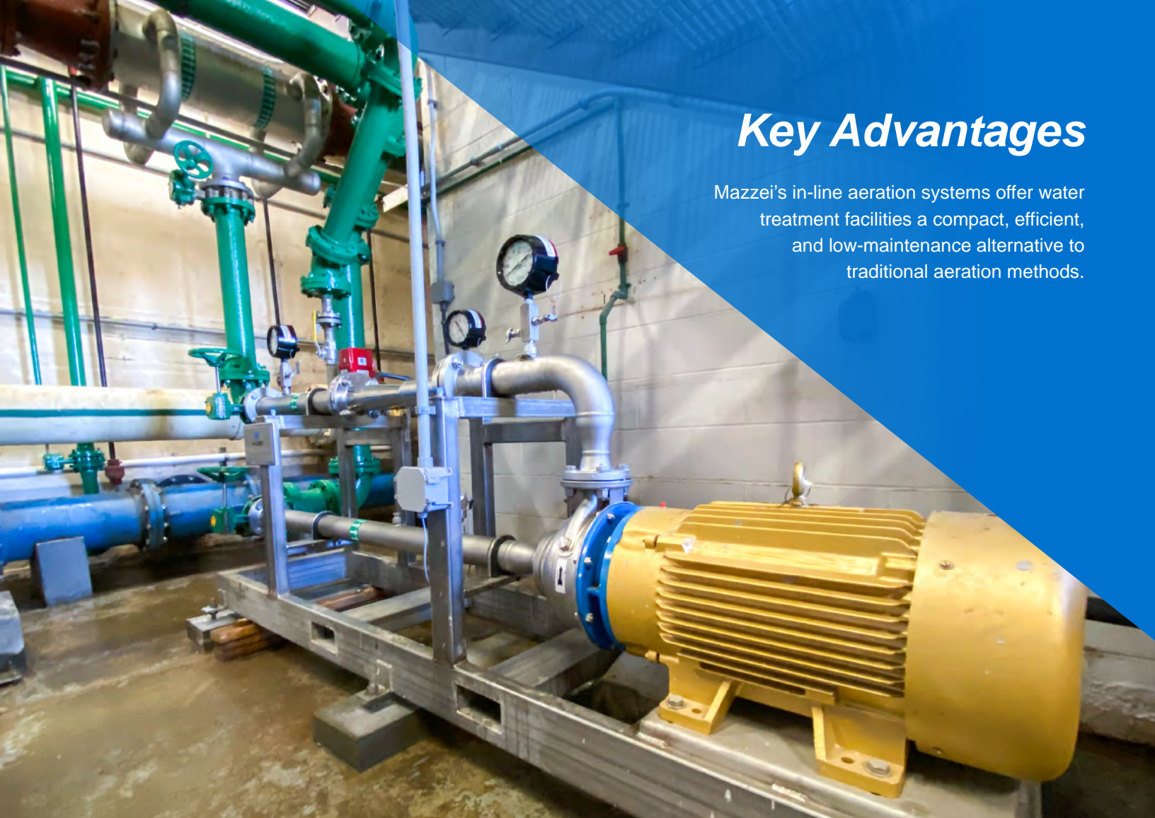
Installation Photo: PFR can be seen installed on mainline in upper left corner; Injection Skid in the foreground.
