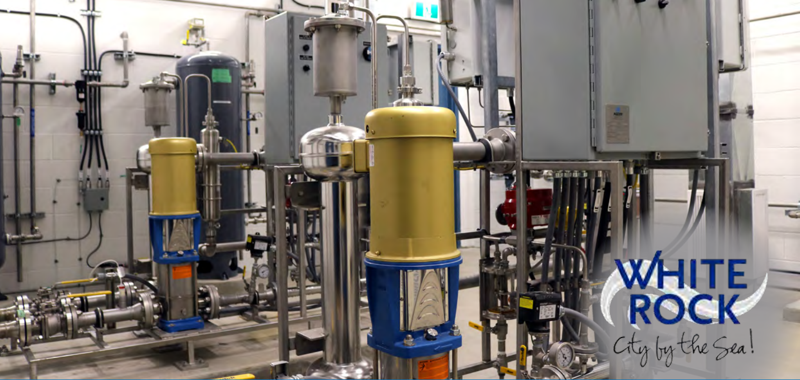
Sidestream Injection Skids
