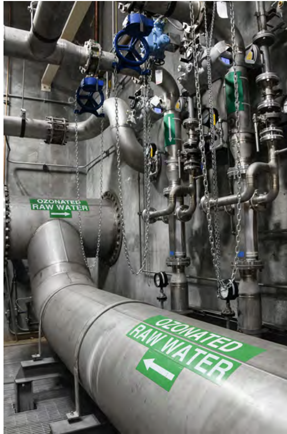
The Mazzei sidestream ozone injectors at Robert A. Duff Water Treatment Plant are going strong 20 years after installation, with no need to replace them during the recent ozone generator upgrade.
