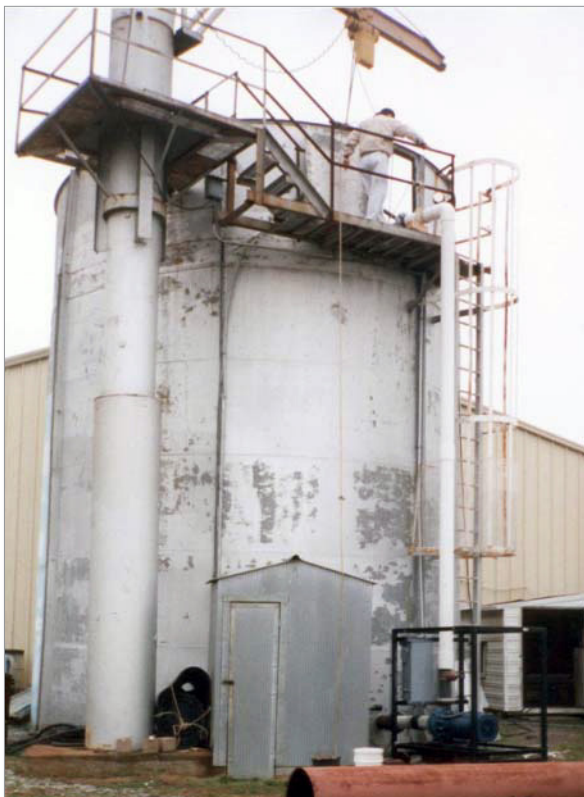
Test tank 21' diameter x 30' deep and a circulation pump
