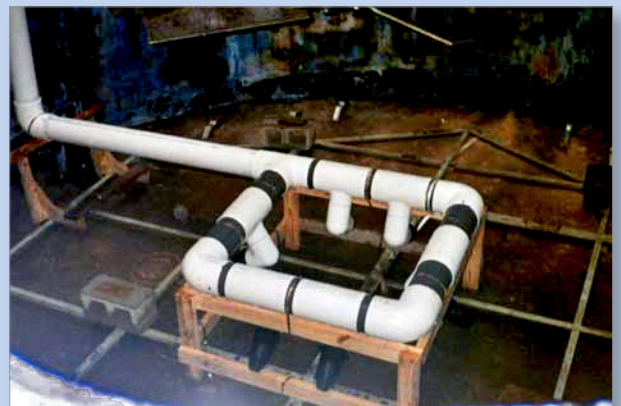
Mazzei N45 nozzles and manifold
