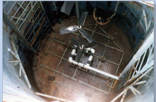
Mazzei N45 nozzles and manifold
