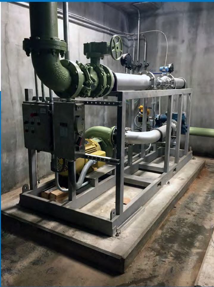
Air Injection Skid
