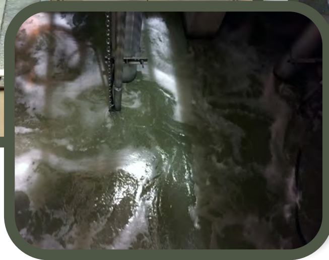
Mixing in basin
