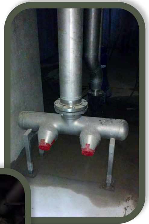
Basin nozzle manifold
