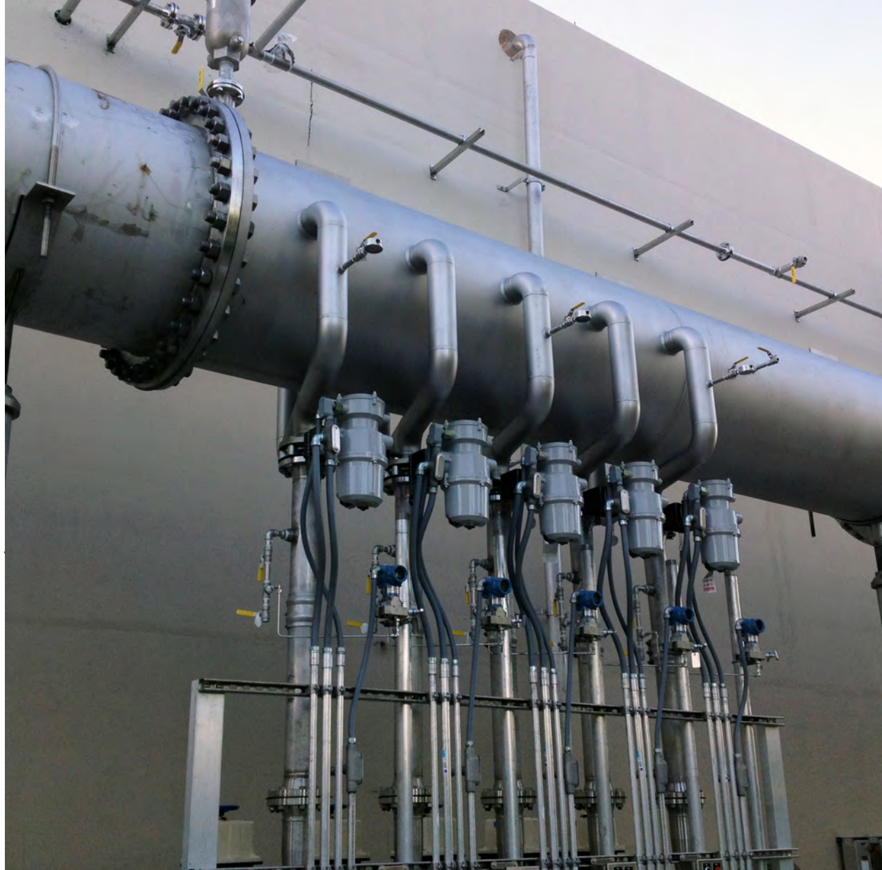
Five venturi injectors ozonate a sidestream flow and mix the treated water into the main flow in a Pipeline Flash Reactor (PFR) at OUC Southwest WTP.
