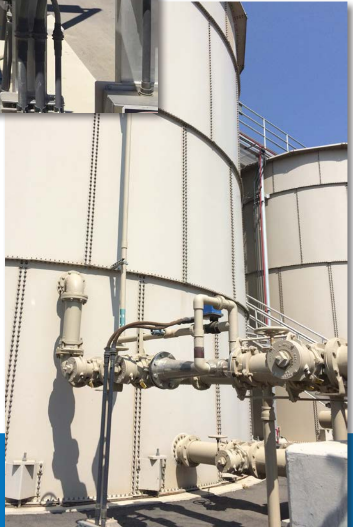
Reedley Wastewater Treatment Plant
