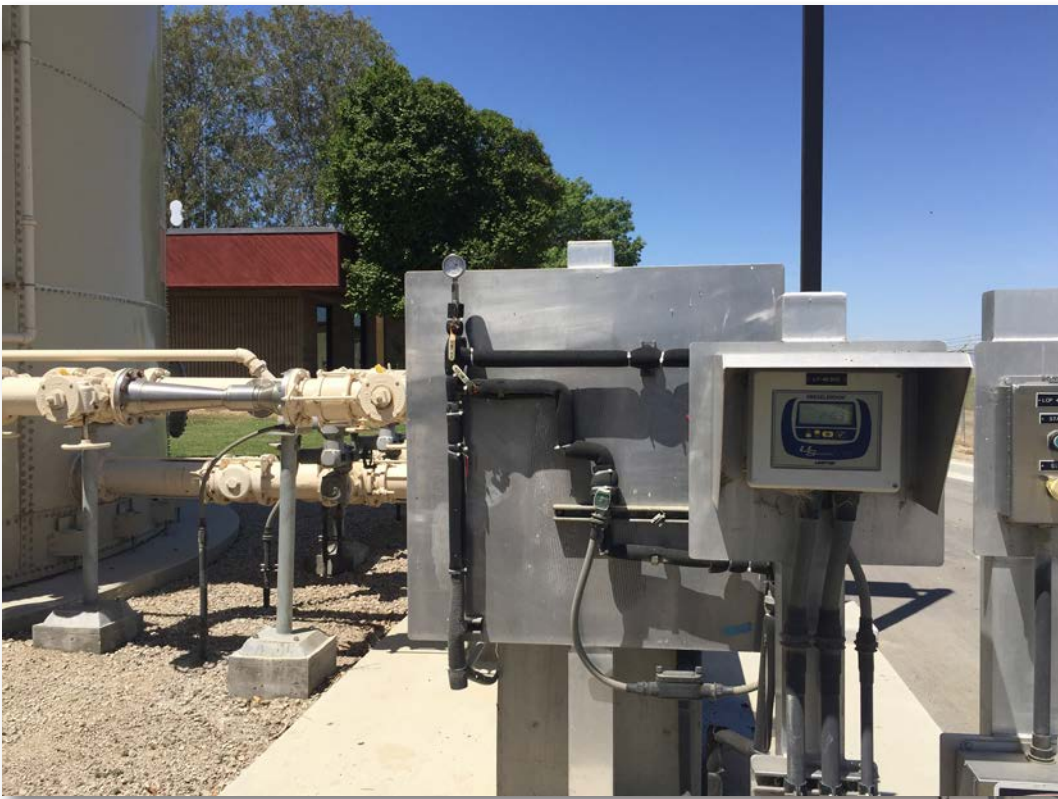
Delano Wastewater Treatment Facility
