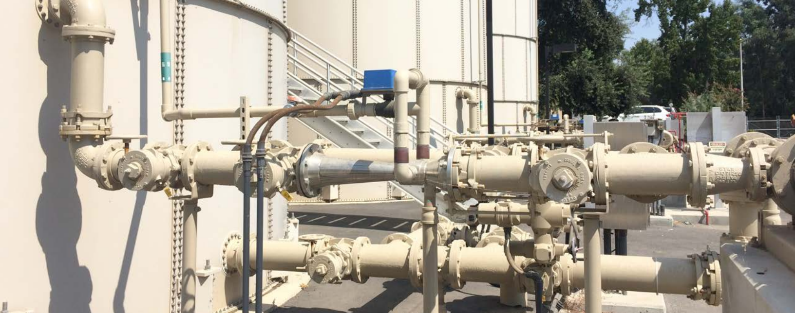
Reedley Wastewater Treatment Plant
