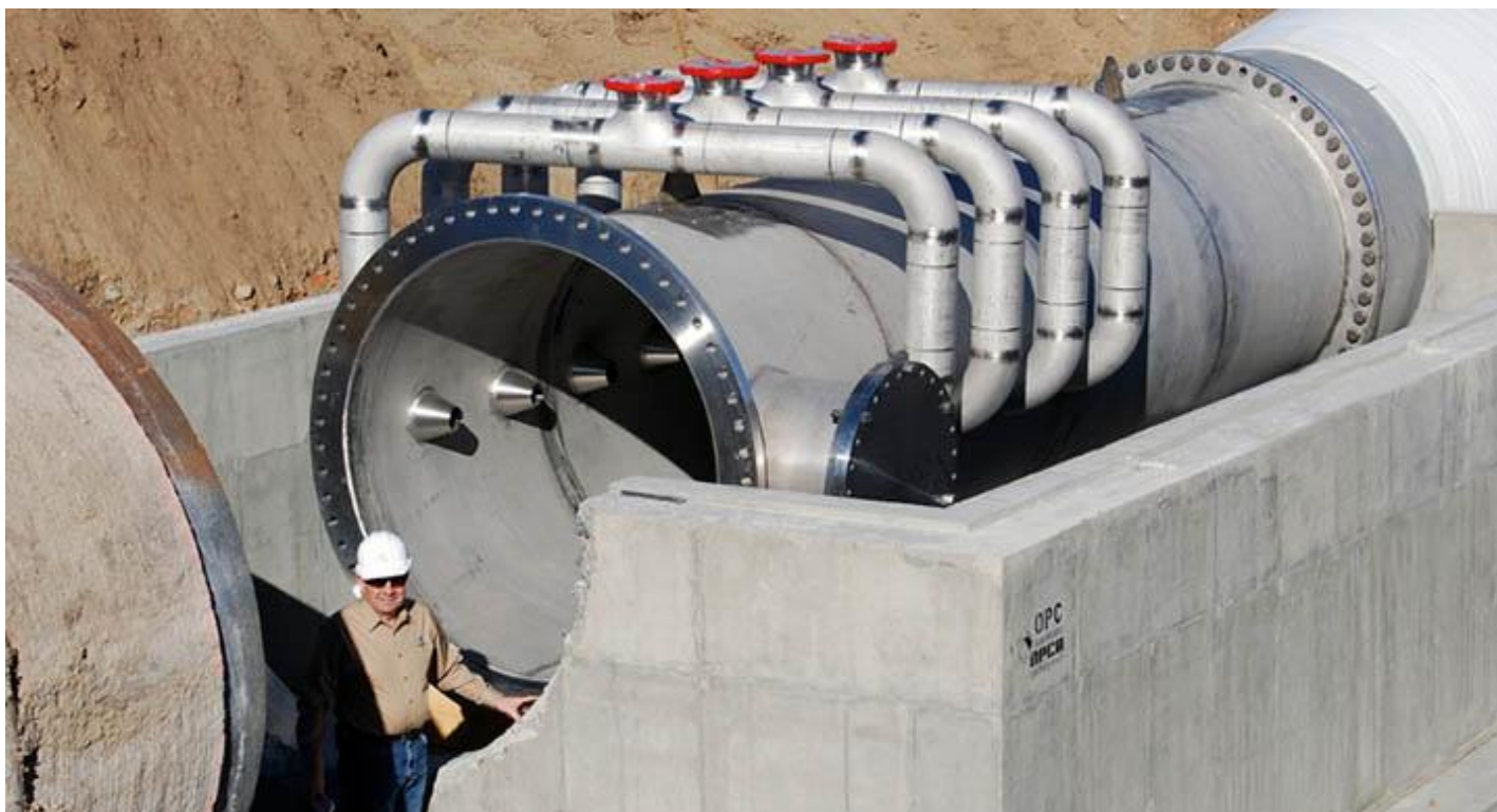
Angelo Mazzei beside a pipeline flash reactor (PFR) at a 140 MGD water treatment plant in Castaic, California. In a short section of pipeline, specially engineered and oriented mixing nozzles blend ozonated sidestream into the main flow.
