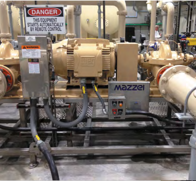
FIGURE 2. GDT/PFR System Control Panel
