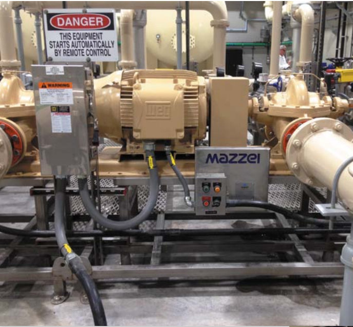
FIGURE 2. GDT/PFR System Control Panel
