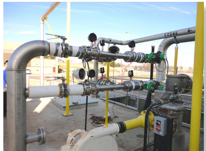
FIGURE 4: Contactor Number 3 ozone injectors
