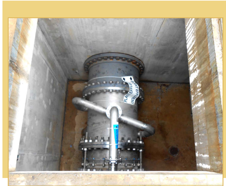
36" Pipeline Flash Reactor
