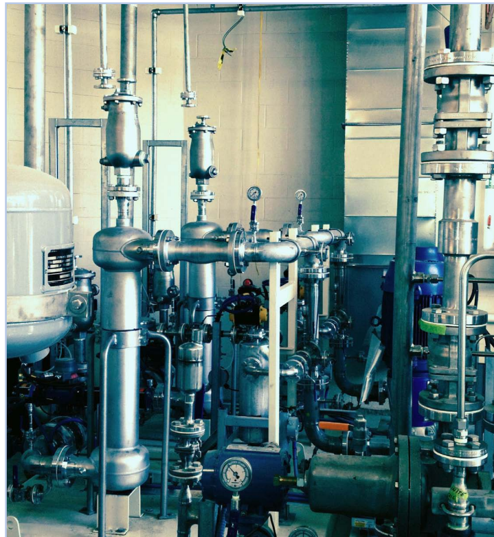
FIGURE 1: GDT Ozone Contacting Skids at Buckingham WTP
