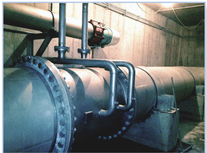
FIGURE 2: PFR at Buckingham WTP
