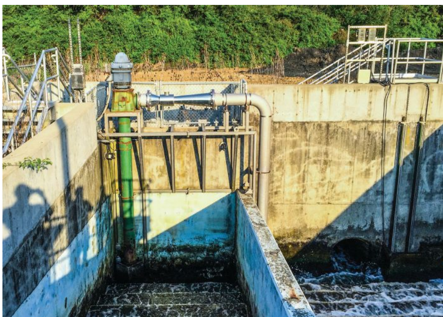
Image 1. This compact aeration system enables municipal wastewater plant to meet and maintain the required dissolved ozone levels during storm events. (Images courtesy of Mazzei)
