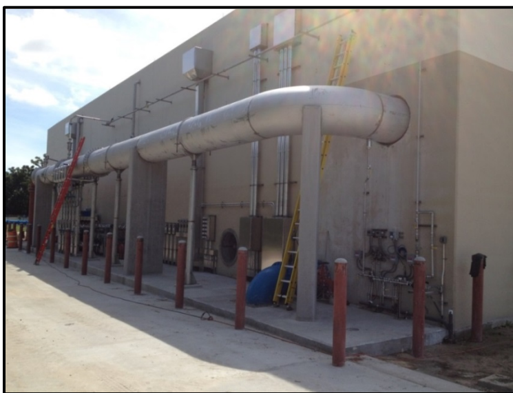
Figure 1. Installation at OUC Southwest plant.
